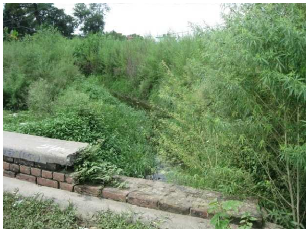
Fig No. 54:- Distributory is full of weeds, shrubsand domestic refuges instead of water supply at Jail Road
